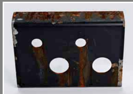
Significant rusting and blistering as well as delamination of primer
